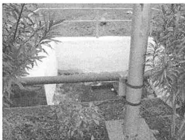
Drain Water Harvesting Pit
