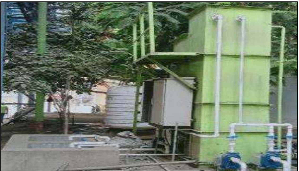
Sewage Treatment Plant Installed at CCR Area
