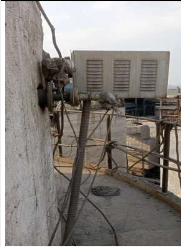
Captive Power Plant
