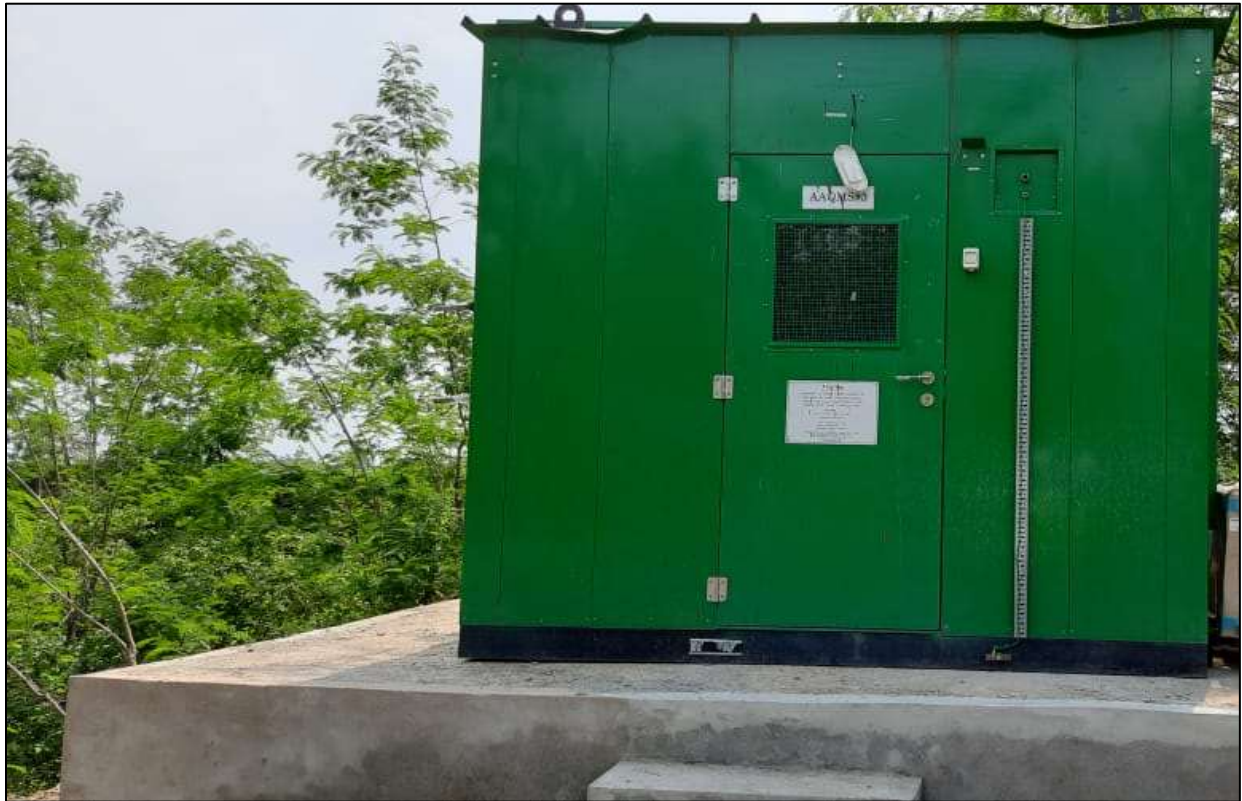
CAAQMS -03 Installed at Crusher Area (Mines)
