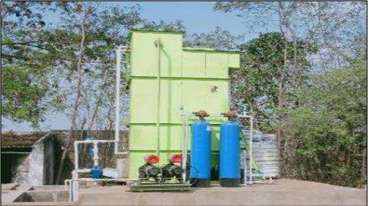
Sewage Treatment Plant Installed at Packing Plant Area
