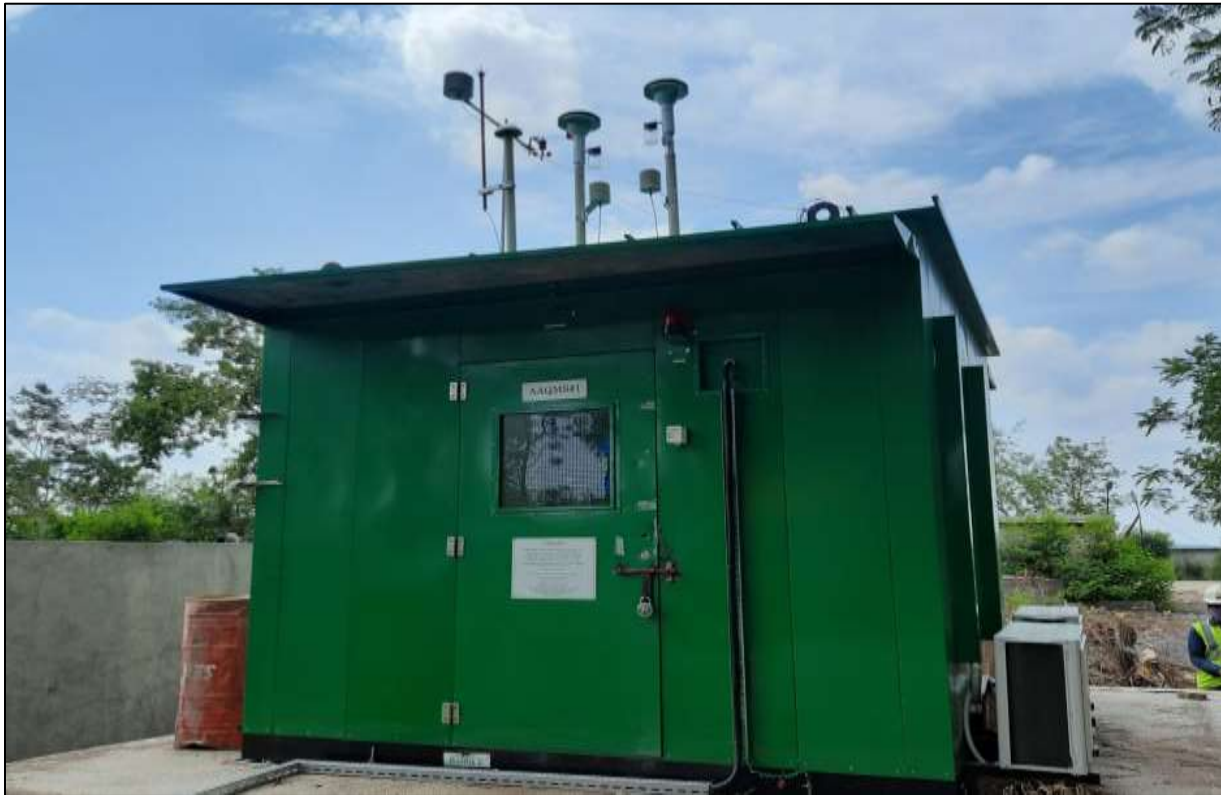
CAAQMS -01 installed at Plant Main Gate
