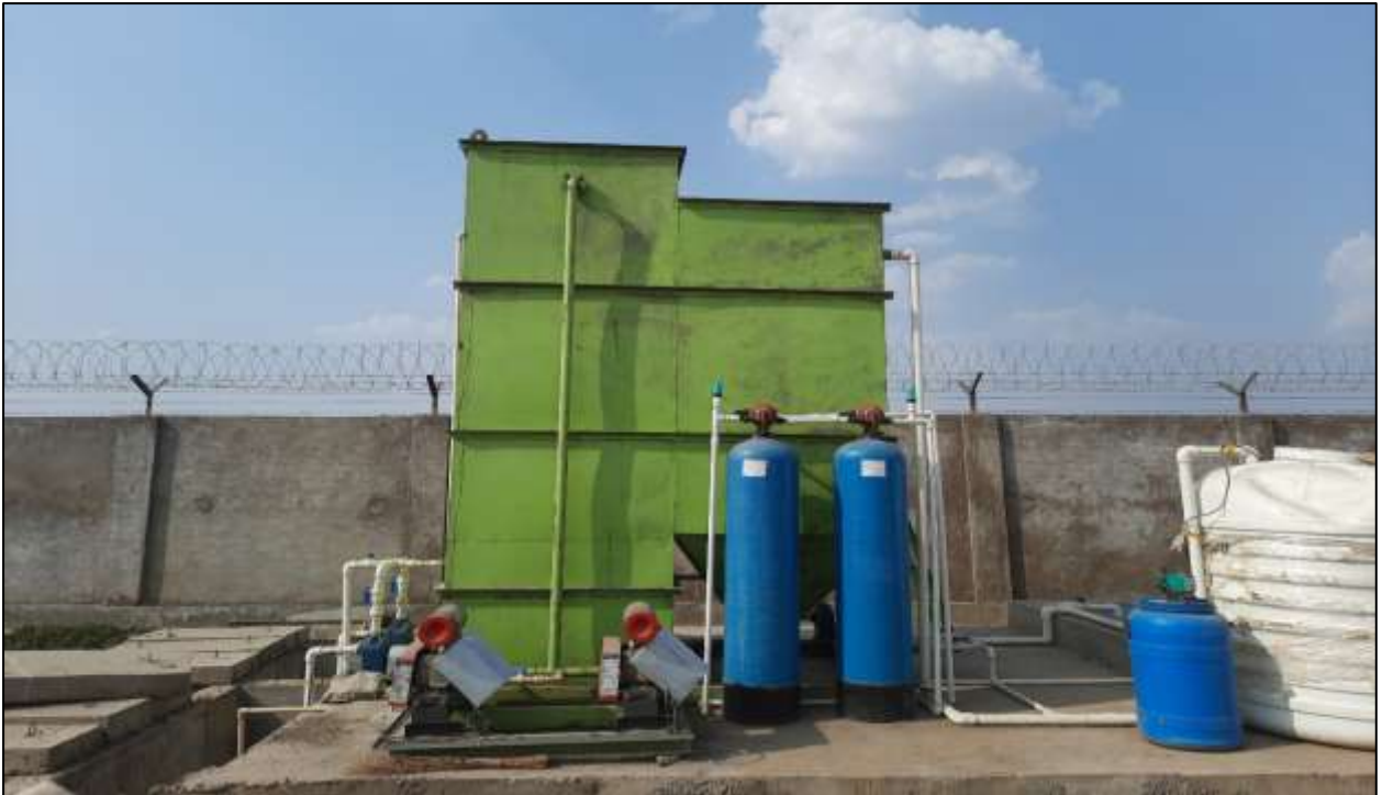
Sewage Treatment Plant Installed at Temporary Hutment Area
