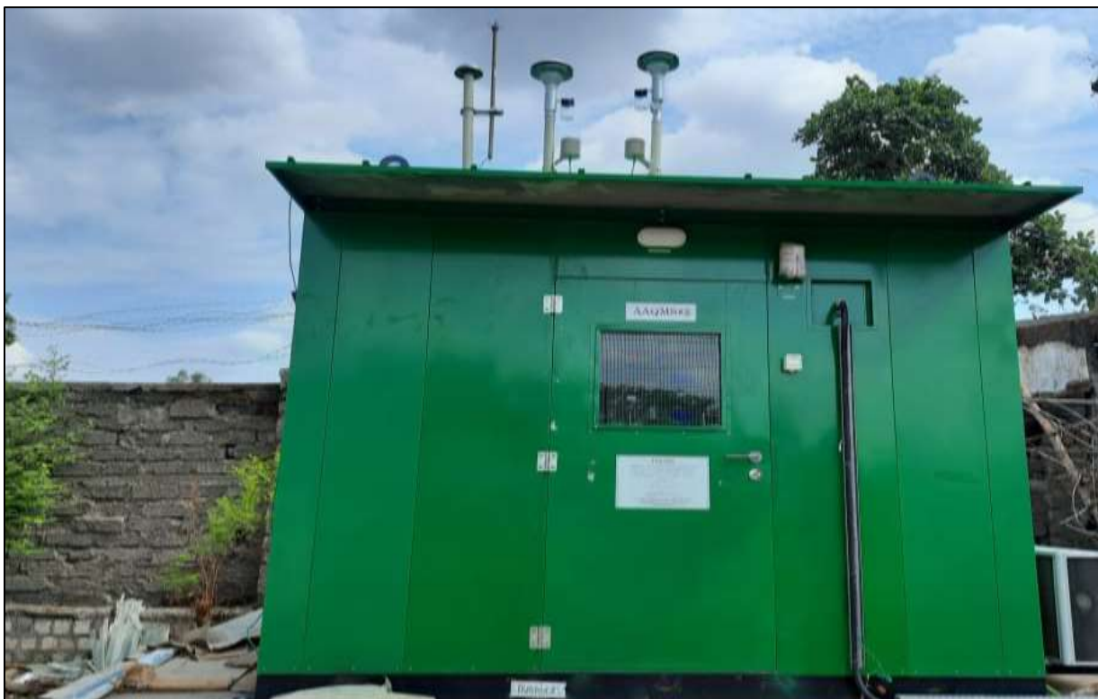
CAAQMS -02 installed at CPP Area
