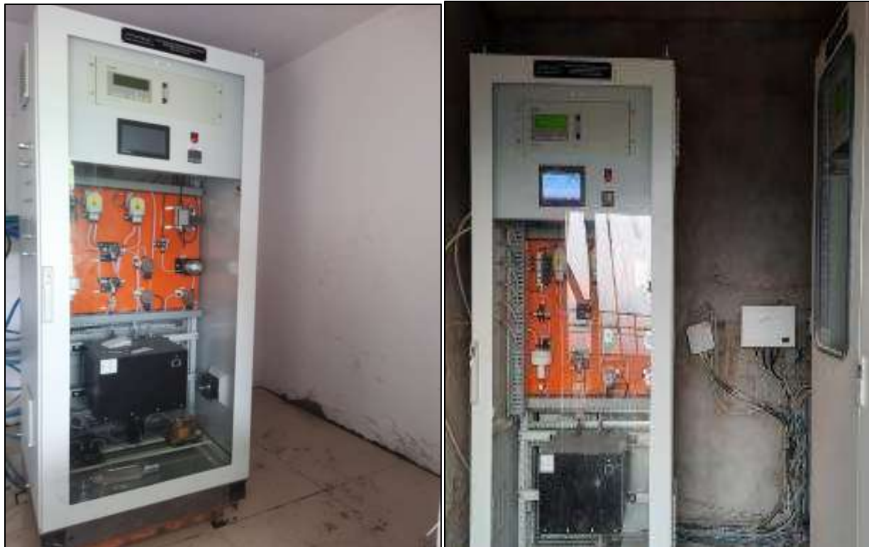
Installation of CEMS for Gaseous Emission Monitoring at Raw Mill + Kiln and CPP
