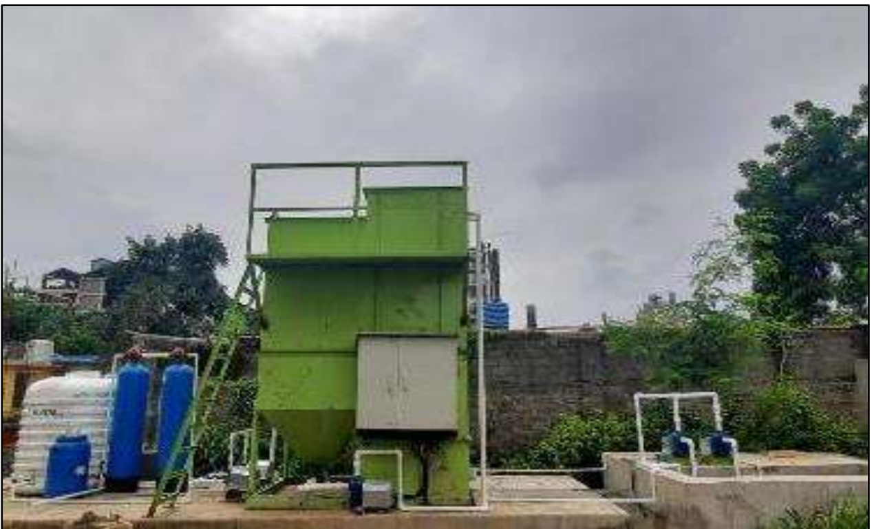
Sewage Treatment Plant Installed at Admin Building Main Gate
